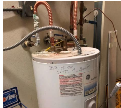
Figure 7: Uninsulated copper DHW pipes
