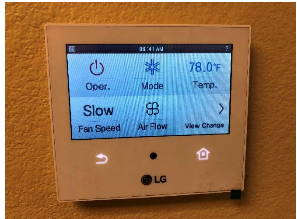
Figure 4: Existing Smart Thermostats in ATCT
