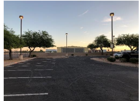
Figure 1: Exterior HPS Fixtures in Parking Lot
