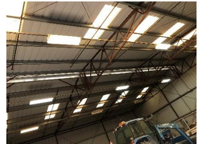
Figure 1: Interior Linear Fluorescent Fixtures
