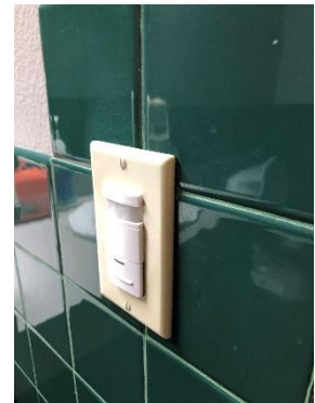
Figure 3: Occupancy Sensor in the Restroom
