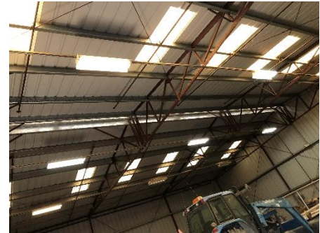
Figure 2: Linear Fluorescent Fixtures in the Maintenance Building
