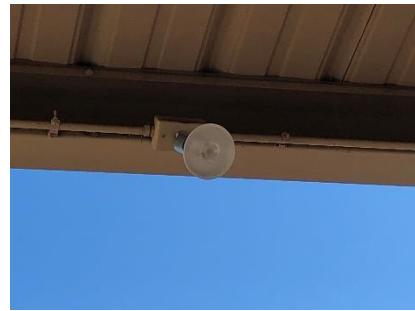
Figure 2: Existing Canopy Lighting Fixtures
