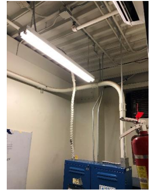
Figure 2: Lighting Fixture in Electrical Room
