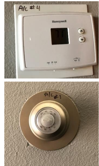
Figure 5: Thermostats in Administration Building
