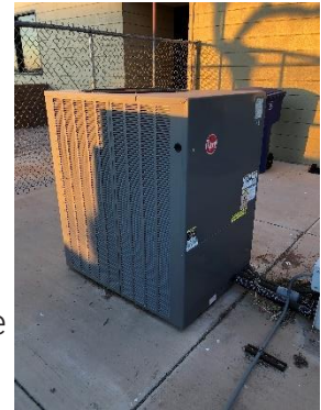
Figure 6: One of four Condenser Units serving the Admin Building
