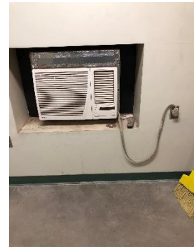
Figure 6: Window Unit in ATCT
