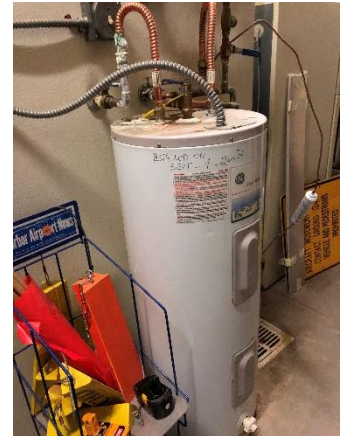
Figure 8: 30 gal DHW Storage Tank
