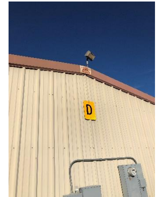
Figure 2: Exterior Halide Fixture
